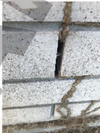
Example of active Termite workings leading into wall cavity.
