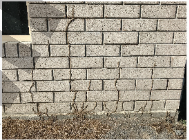
Example of active Termites to front wall of House.
