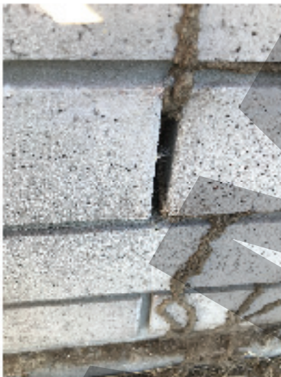
Example of active Termites to front wall of House.
